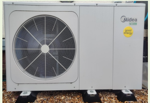
Heat Pump on the Patio of Ian and Charlotte's House
