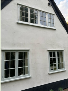
Old Single glazing (ground floor) vs. New Heritage Slimline double glazing (1st floor).
