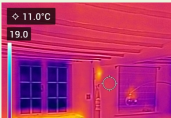
Thermal image of heat loss through window on the left (purple), slightly reduced by the existing blind (right)
