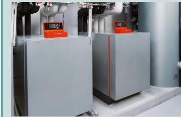
Ground Source Heat Pump
