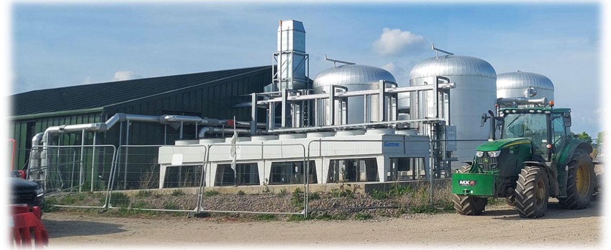
Swaffham Prior Heat Network – Energy Centre (Equans)
